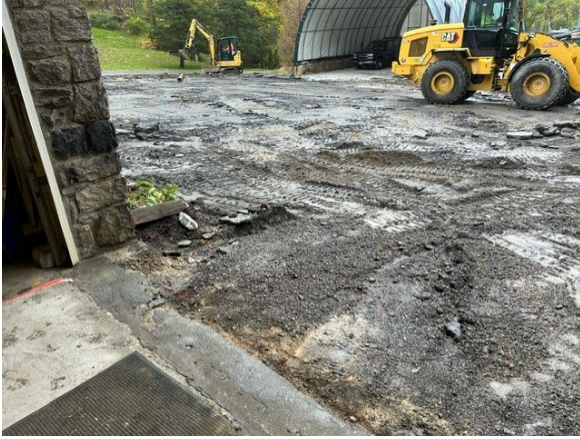
Image 5: Damage outside Ludington Court Highway Garage in July 2023 in Kent, NY | Kent Highway Department.
