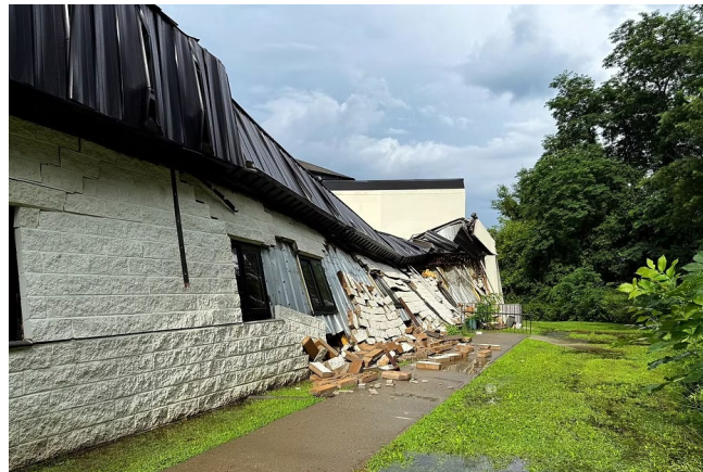
Image 2: Damage to Hudson Valley InterArts building in Patterson following a rain event in July, 2025 | Patterson Fire Department, accessed via Putnam County Times & Putnam County Press
